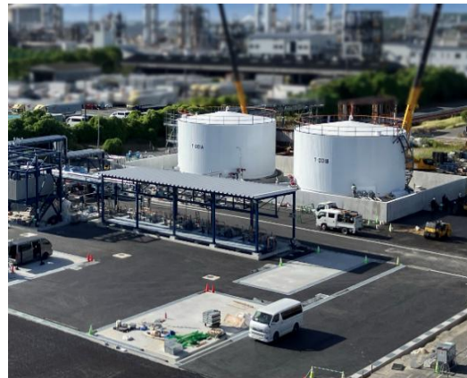
Facility for receiving used cooking oil as feedstock for SAF (on the premises of Cosmo Oil's Sakai Refinery)
