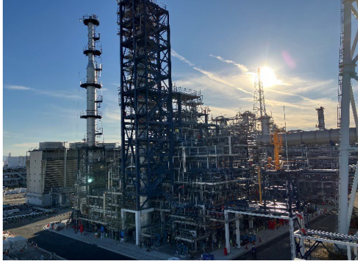
SAF production line under construction (on the premises of Cosmo Oil's Sakai Refinery)
