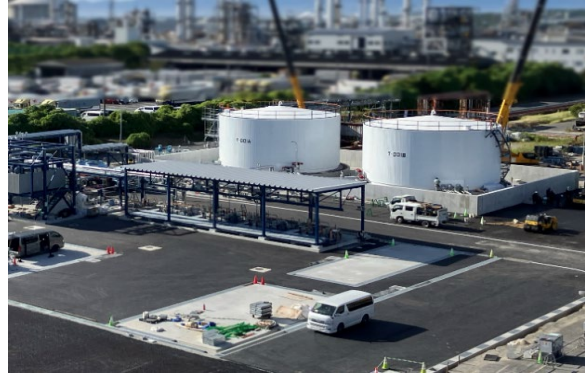
Facility for receiving used cooking oil as feedstock for SAF (on the premises of Cosmo Oil's Sakai Refinery)
